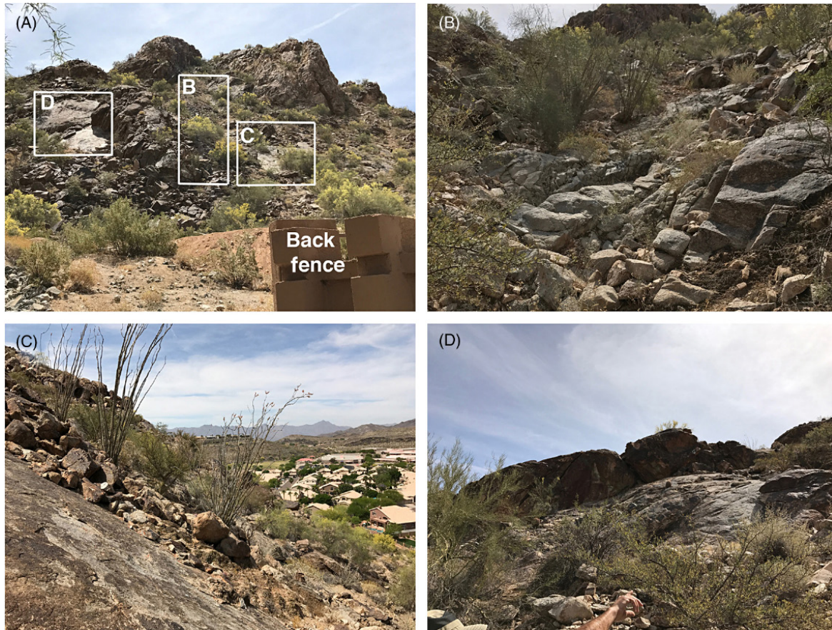
FIGURE 10.14 (A) is from the perspective of looking at the mountain slope from the resident's back fence, where (B) debris flow levees, (C) talus from rockfalls, and (D) a rockslide all represent hazards above a suburban neighborhood. Note the massive rock in (D) that is situated on the pressure-release joint of granitic surface with little to no support to inhibit the next mass-wasting event.
