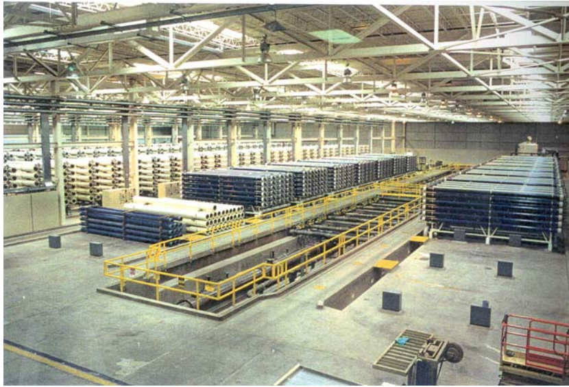
Figure 3.7 Yuma Desalting Plant Process Area. Pressure vessels for the 8-inch reverse osmosis elements.
