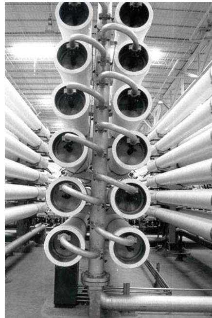
Figure 3.9 Control Block at the Yuma Desalting Plant. Bank of pressure vessels that hold reverse osmosis elements in the process area.
