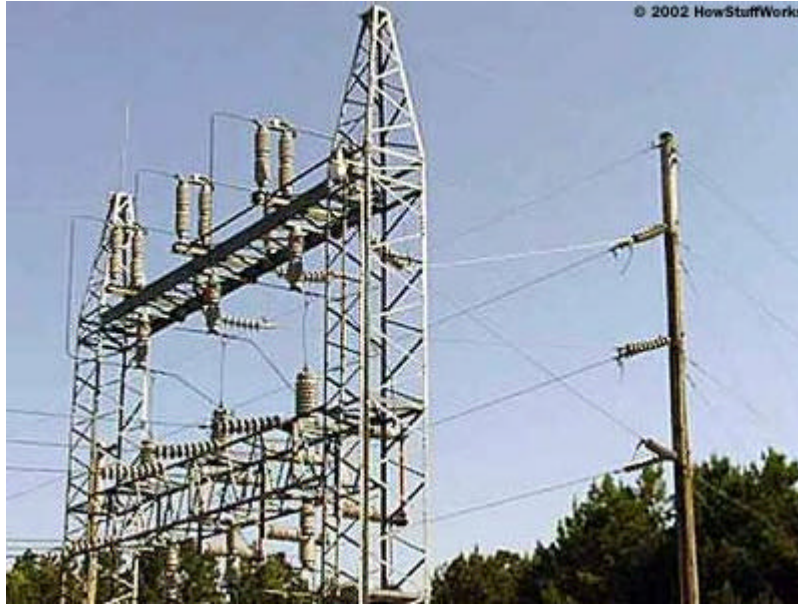
The transmission lines entering the substation and passing through the switch tower
