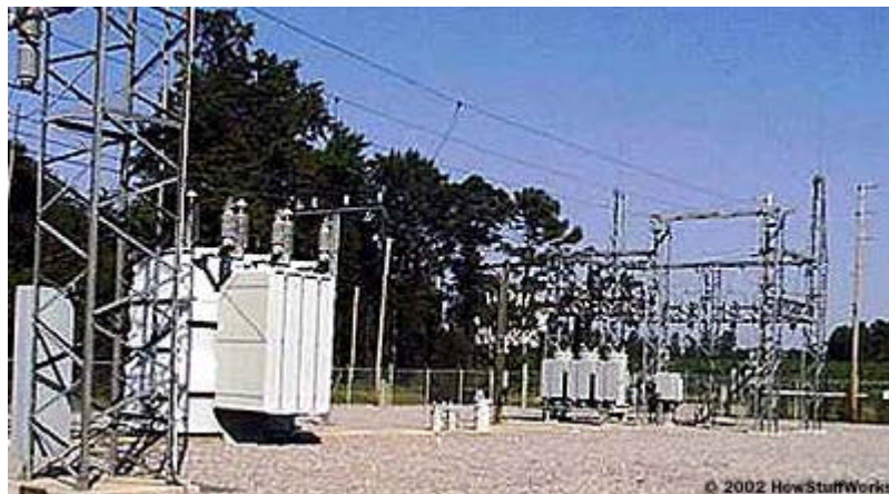
A typical small substation
