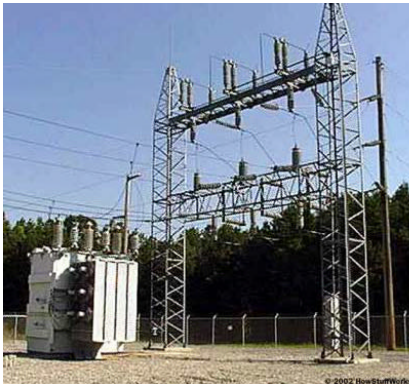
The switch tower and the main transformer
