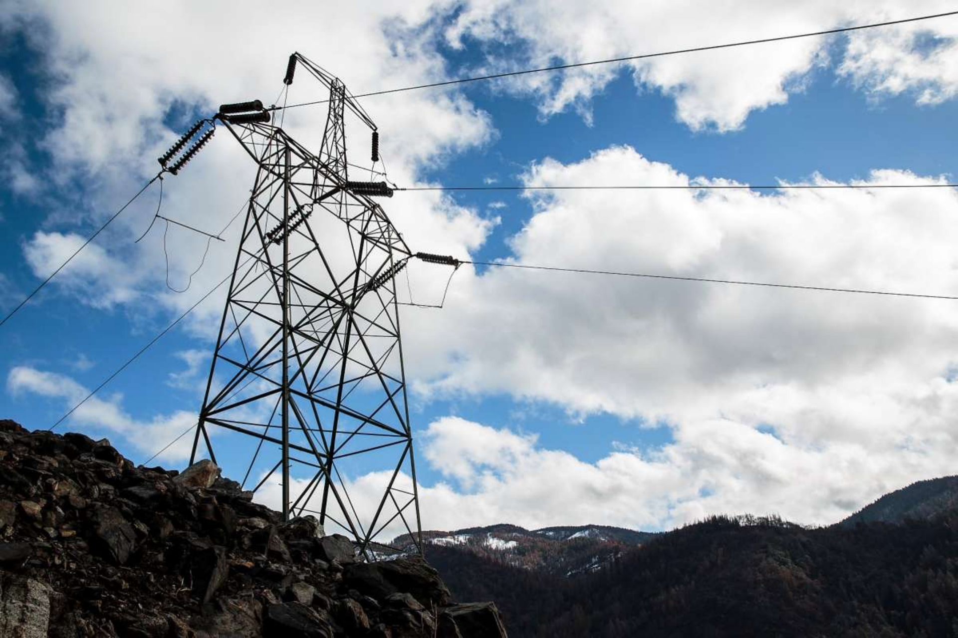
The PG&E transmission tower that sparked the Camp Fire, in Pulga, Calif., Feb. 28, 2019. | Max Whittaker / The New York Times
