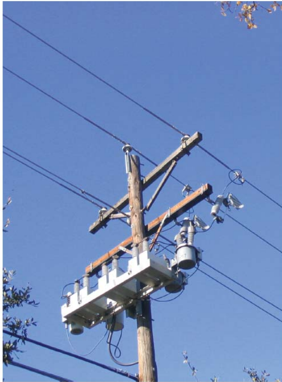
Figure 1.11 Pole-mounted three-phase distribution capacitor bank.
